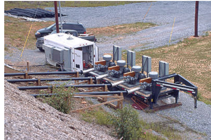
Blower System at Williamson County
